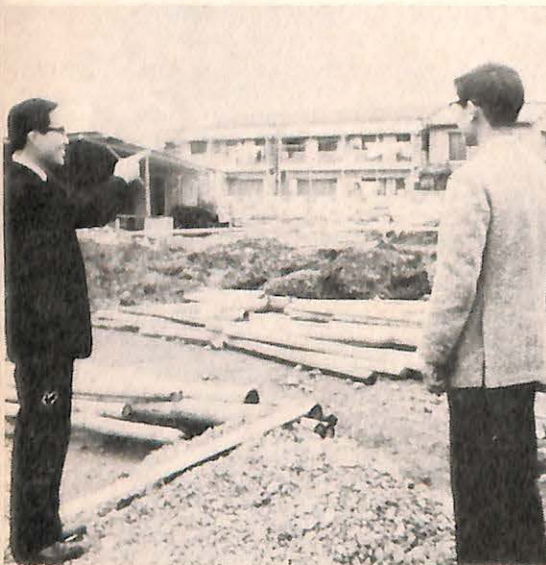
Rev. Hisaschi Murakami and Mr. Fujie, a part-time student at O.B.S., looking at the new dormitory-dining hall of O.B.S. under construction.
