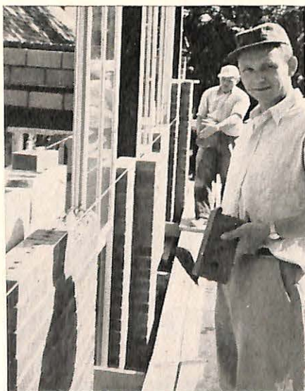
More bricks go into the wall of the German Baptist Mission Church of Hamilton, Ontario.
